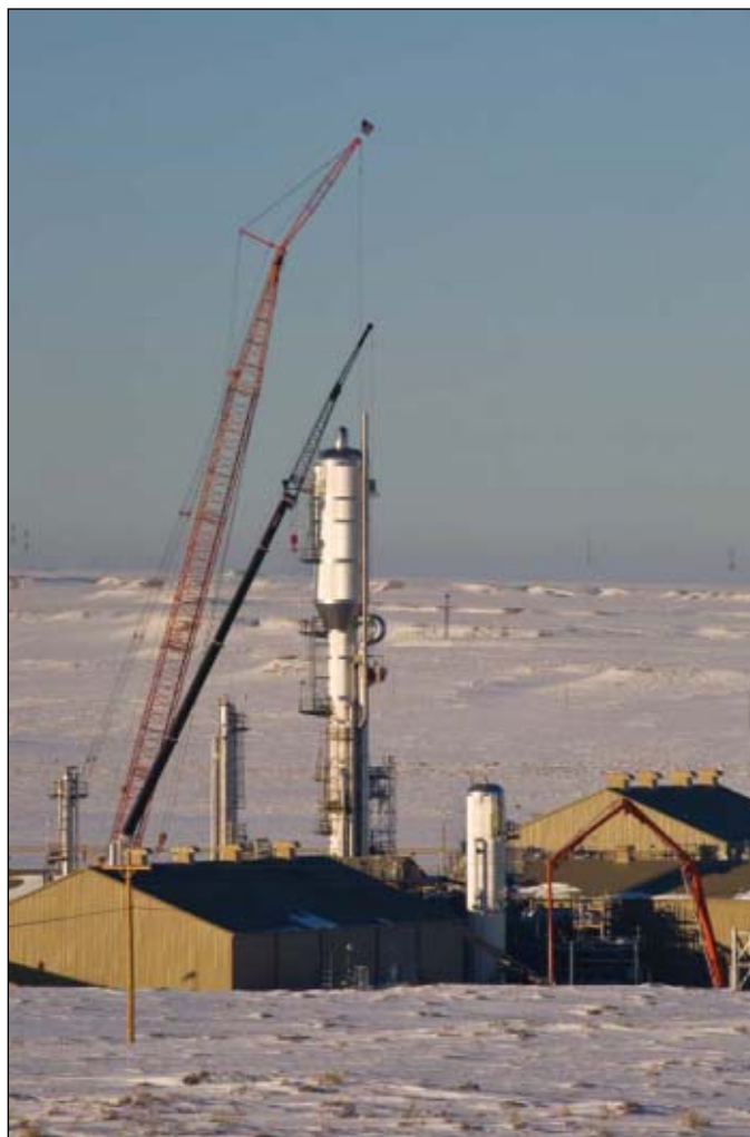
In February 2008, Enterprise Products Partners started up the 750-MMcfd Pioneer gas plant in Sublette County, Wyo., near the Opal hub. Photograph from Enterprise Products Partners LP.
